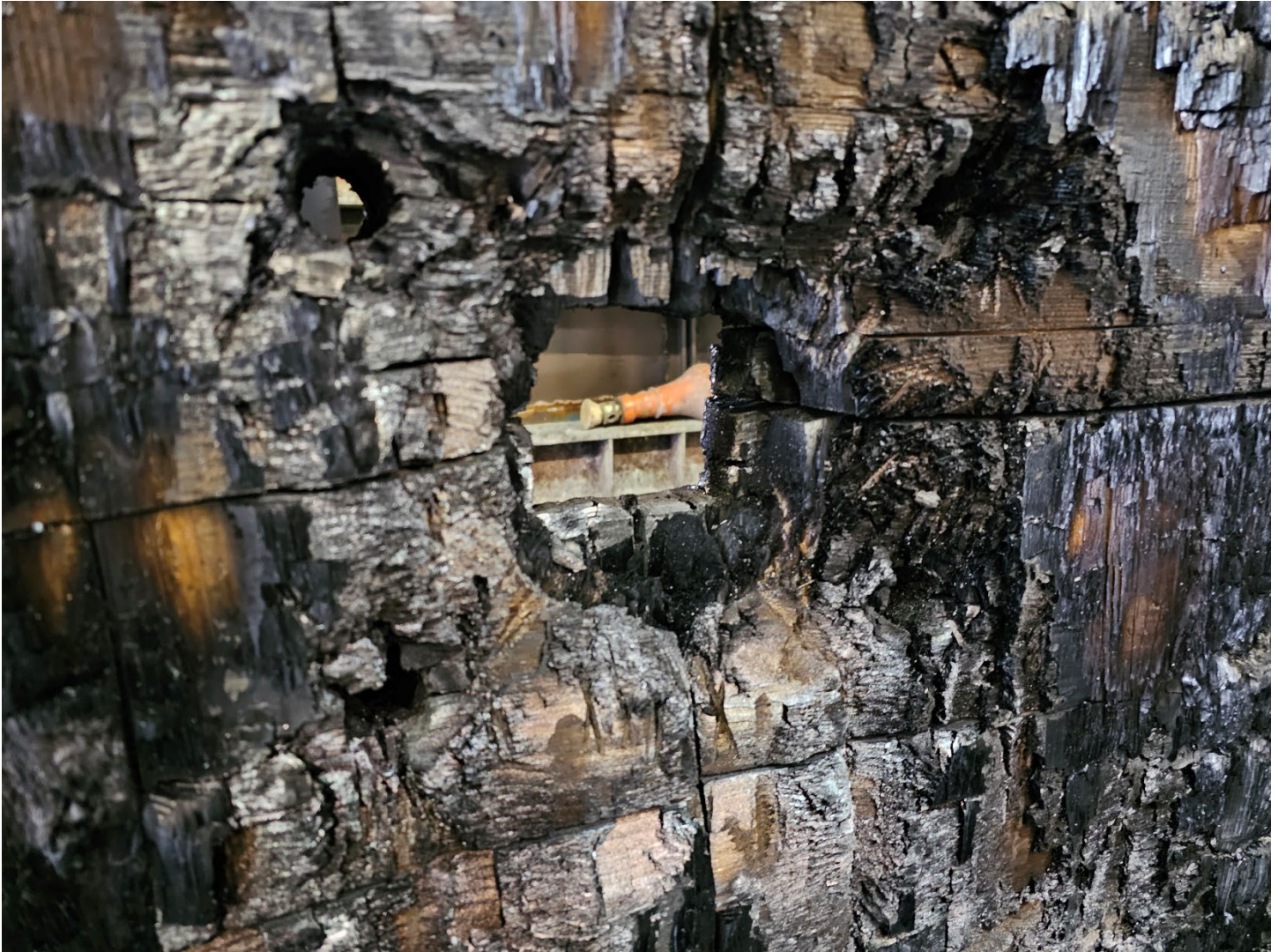
Figure 12. Localized damage through steel column 3 inch x 3 inch steel tube penetration through the CLT assembly.
