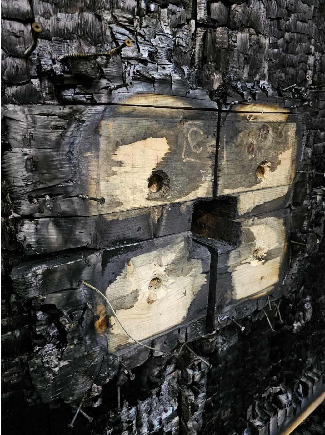
Figure 12: Localized damage through steel column 3 inch x 3 inch steel tube penetration through the CLT assembly.
