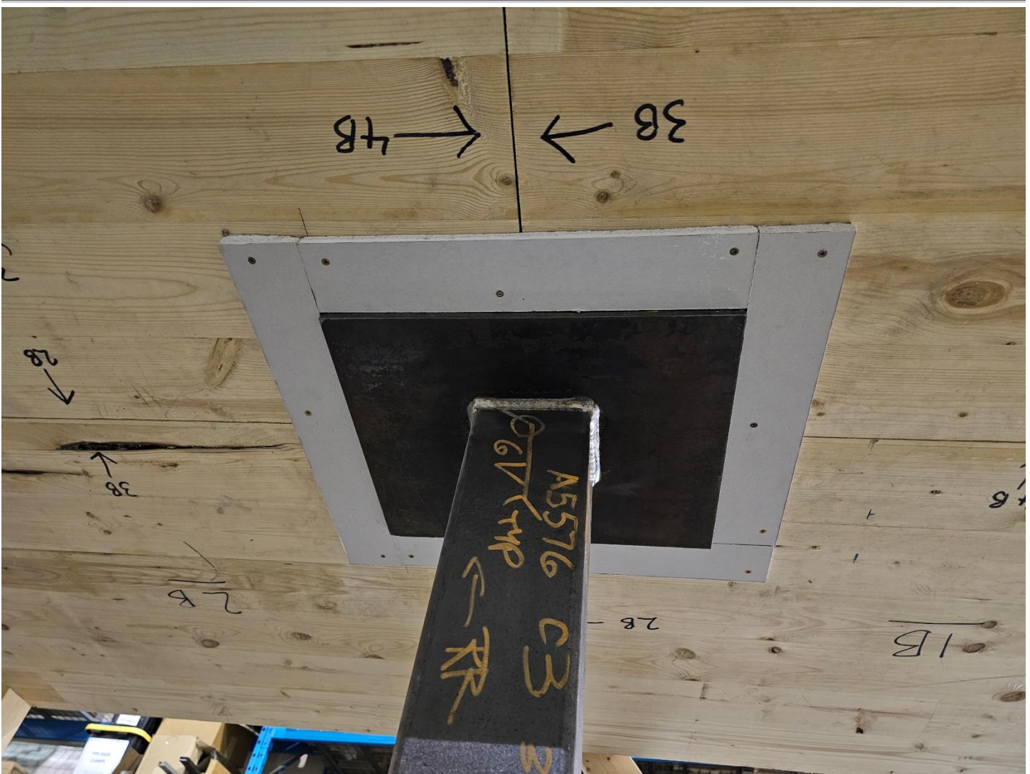
Figure 6: First Layer of Gypsum Board Protection Around Steel Column Lower Plate Connection
