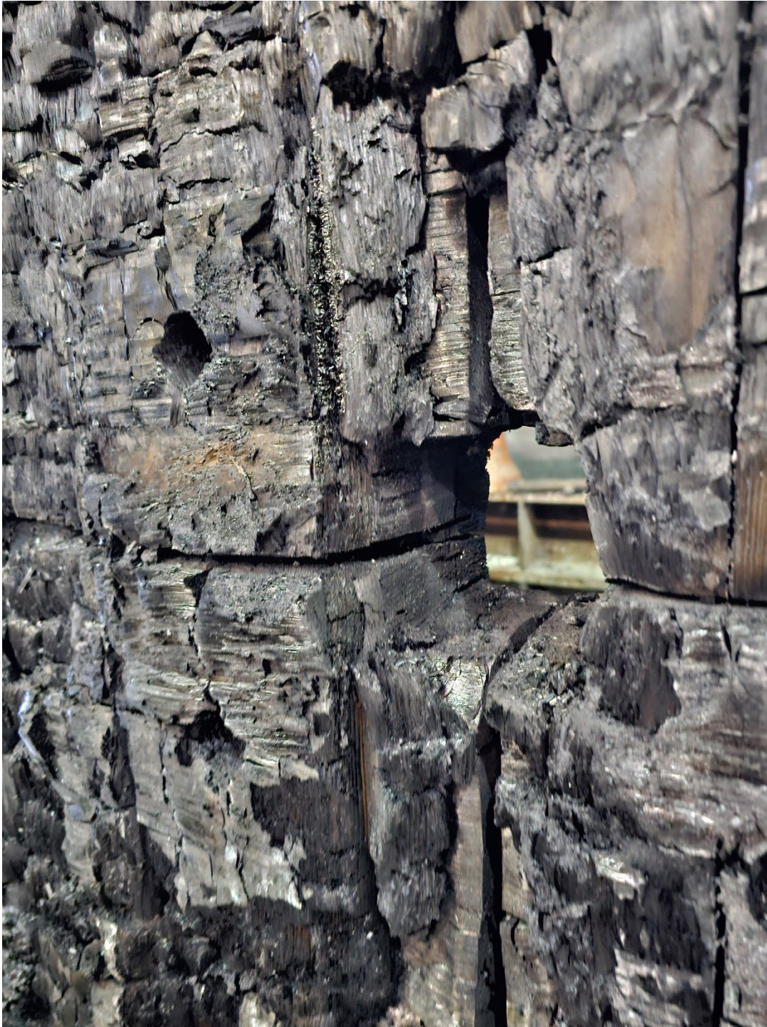
Figure 12. Localized damage through steel column 3 inch x 3 inch steel tube penetration through the CLT assembly.
