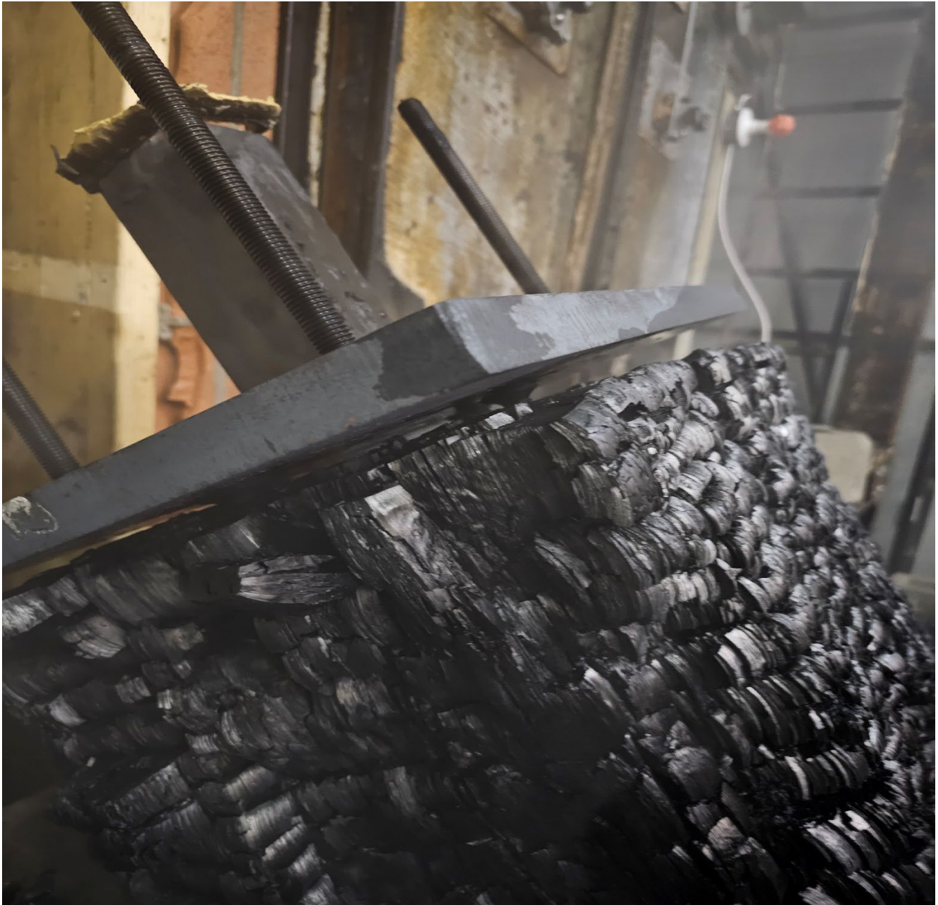
Figure 11. Glulam column retaining steel connection after fire exposure.
