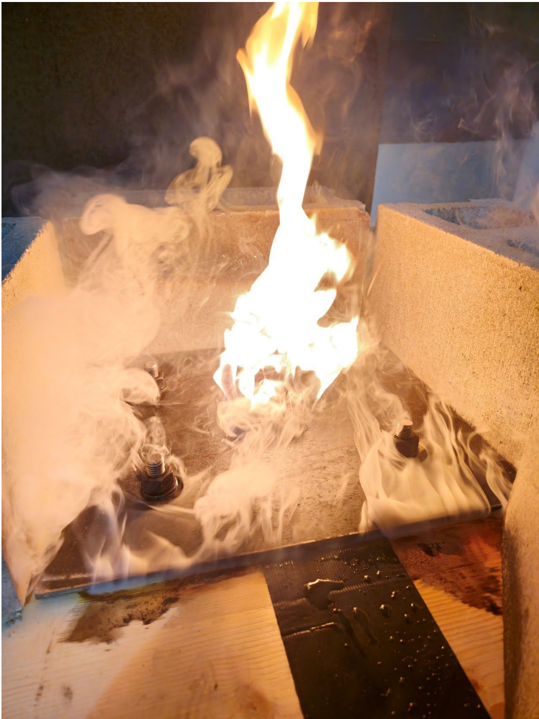
Figure 8: Flaming non-fire side through and around 3 inch x 3 inch steel tube (including concrete masonry weight)
