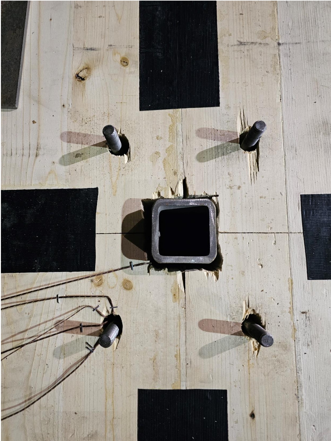
Figure 8: CLT panel joints and steel column connection prior to steel plate installation.
