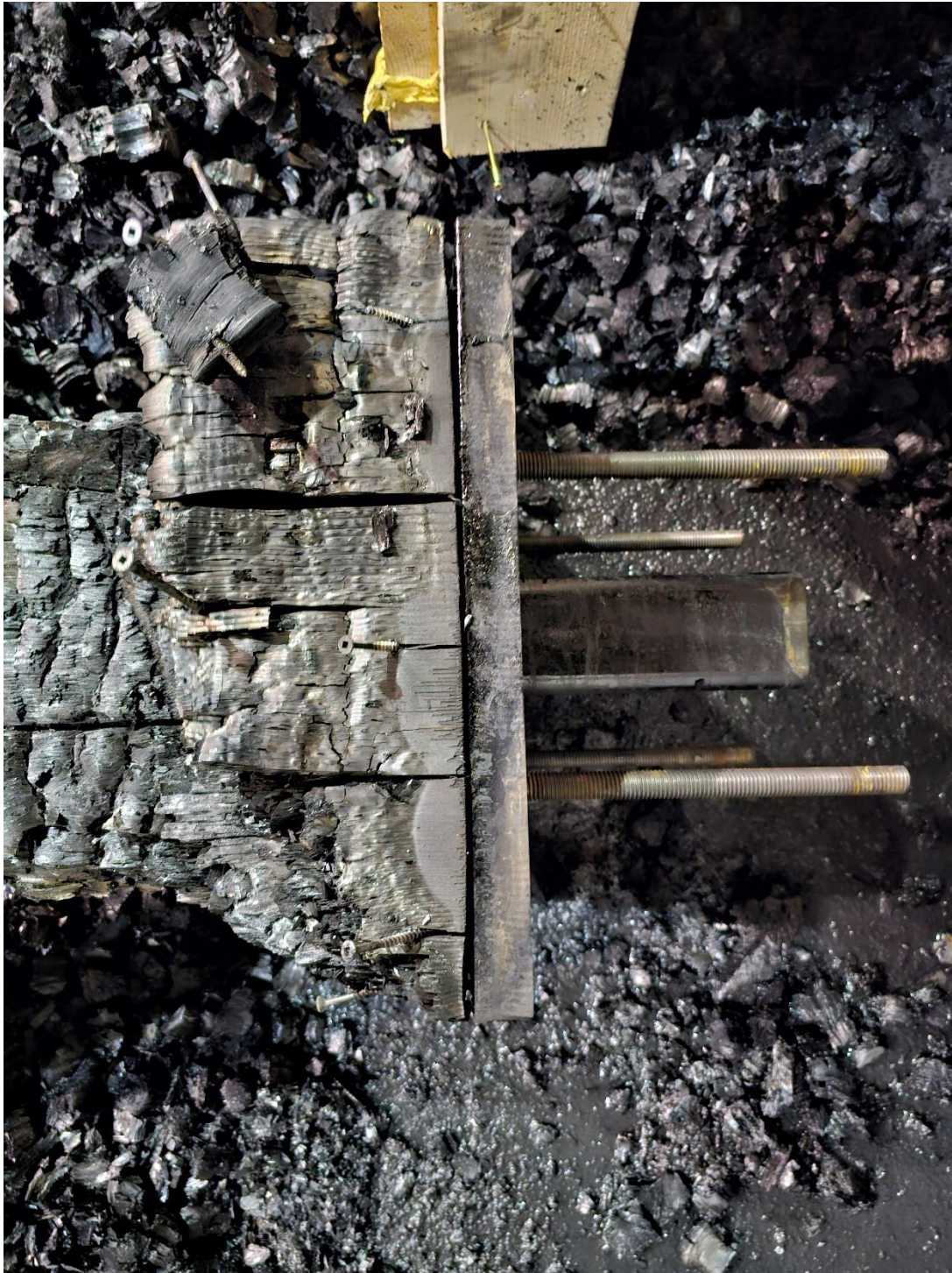
Figure 11: Glulam column and steel connection after fire exposure.
